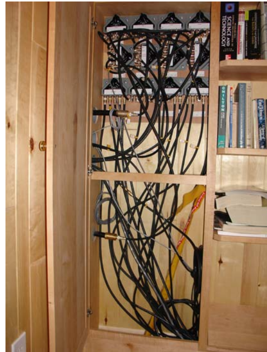
Coaxial cable entry and switching array
