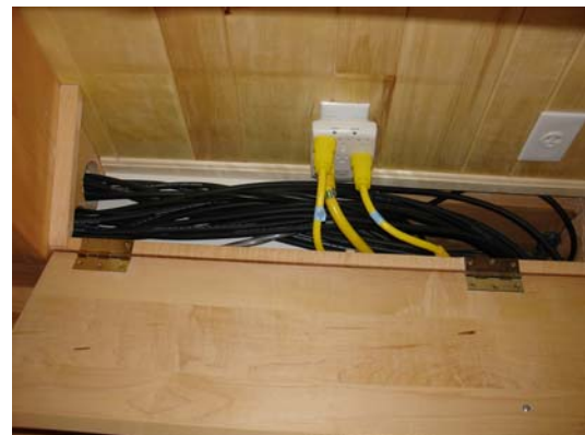
RF and power cable entry underneath the floor
